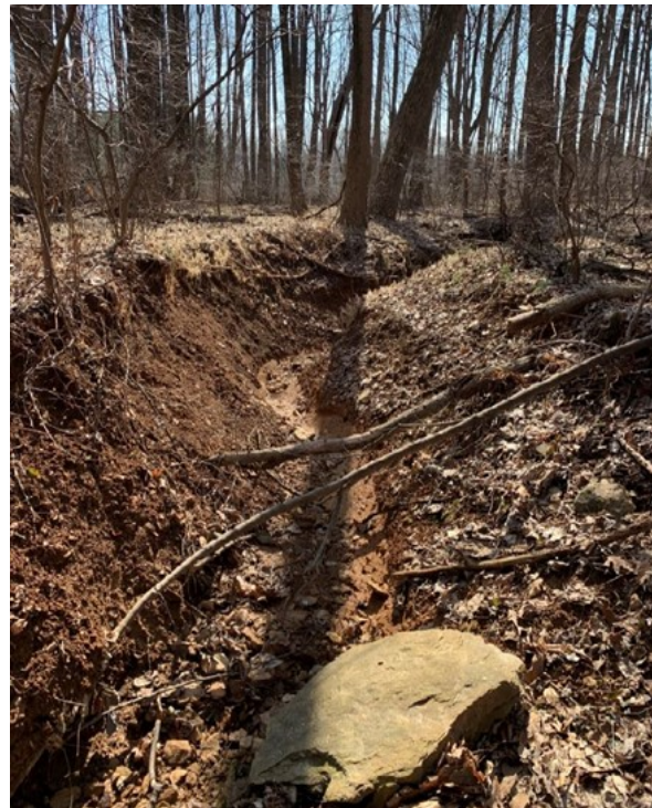
Unmanaged stormwater within this outfall channel has caused major erosion upstream of the Oklahoma restoration project.
